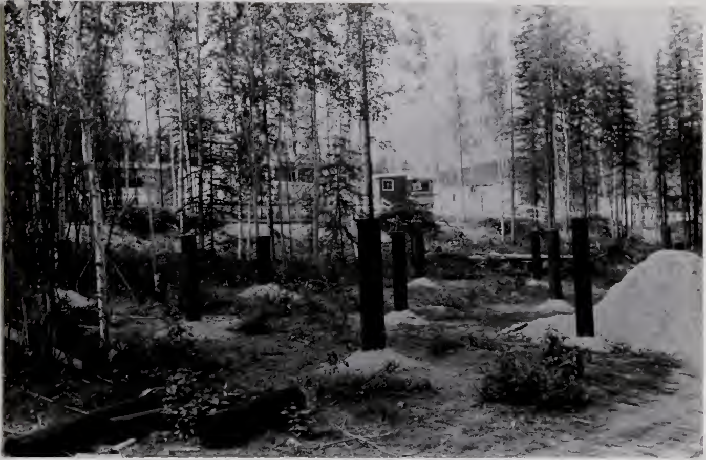
Plate 6. Piles "freezing in" before house construction. Note how many trees have been retained. (July 1970).
